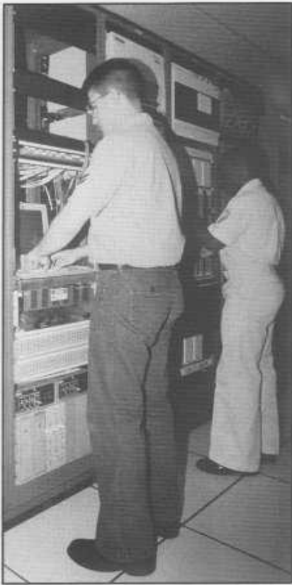
(above left) CTO2 Ben Tomlin and CTOSA Tige Chambers tracking communication circuits through the comm shop.
